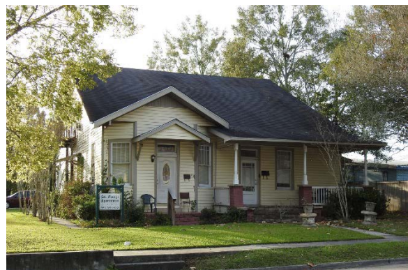
Image 27. A c. 1925 single-family residence at 219 North Florida Street (Survey ID #230). The character of this dwelling's primary facade has been drastically altered by the removal of a dormer, addition of a door opening, and porch modifications. Not only has the integrity of this building diminished, it can no longer be categorized within an architectural style due to the loss of character-defining features.
