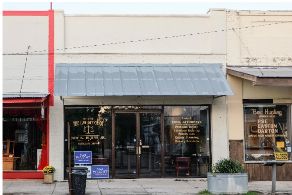
Image 26. A c. 1920 commercial resource at 317 North Columbia Street (Survey ID #304B). The glass double doors and floor-to-ceiling windows on this resource are non-historic additions and have replaced an inset single-door and partial height windows. The scale and materials of the storefront modifications have diminished the integrity of this resource, and it is no longer recognizable as an early twentieth-century Commercial Style building.
