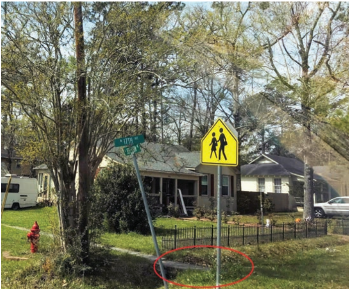
Figure 3.10: Intersection of 17th Avenue and Jefferson Street sidewalks (Source: Digital Engineering; May 2018)
